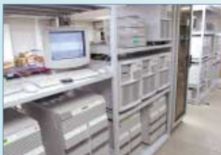
Windows2000 Active DirectoryとExchange2000の導入
